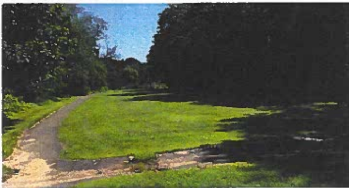
Evidence of ponding at the end of one of the asphalt channels. Water is coming from the forested hill on the right.
