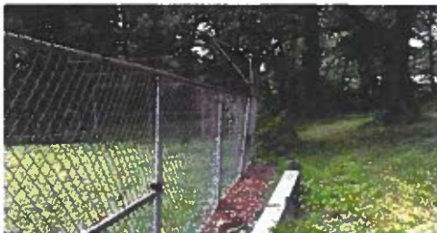
Both baseball backstops at Turner Field are in poor condition and should be removed or replaced.
